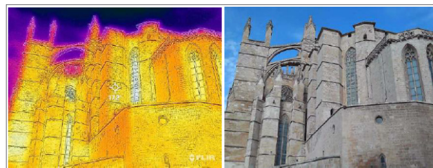
Figure 16: Exterior thermographic analysis of the chevet of the Palma de Mallorca Cathedral (photographs by the author).
