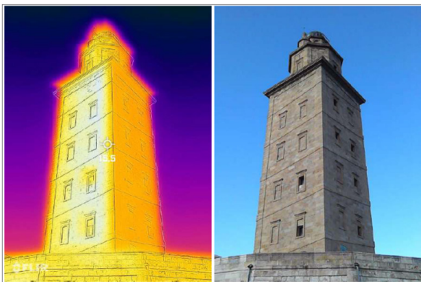
Figure 12: Thermographic analysis of the Roman lighthouse Torre de Hércules, in La Coruña. We can see, on the left, the photograph taken by a thermographic camera and, on the right, the same photograph taken by a photographic camera (photographs by the author).
