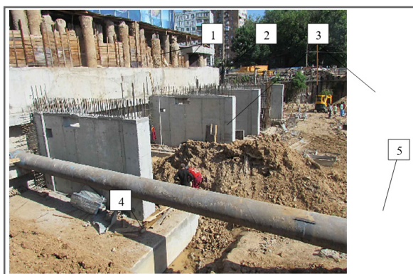
Figure 3: Fragments of completed monolithic reinforced concrete buttresses: 1-existing bored piles to enclose the excavation; 2-fencing of the pit from monolithic reinforced concrete; 3-monolithic reinforced concrete buttresses to reinforce the existing retaining wall; 4-monolithic reinforced concrete grillage; 5-existing pipe - amplification shooting.
