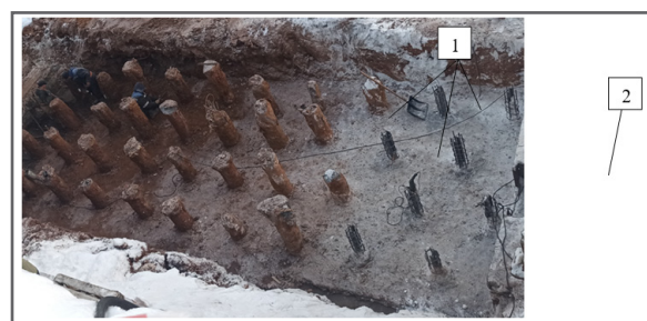
Figure 2: Pile field for a monolithic reinforced concrete buttress: 1-heads of EDT bored injection piles; 2 - concrete preparation for grillage.
